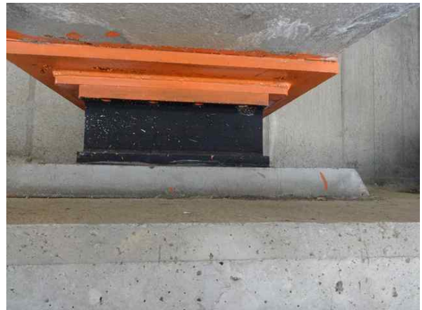
A1-Sh3 무수축몰탈 균열 (0.2mm/0.1m)
