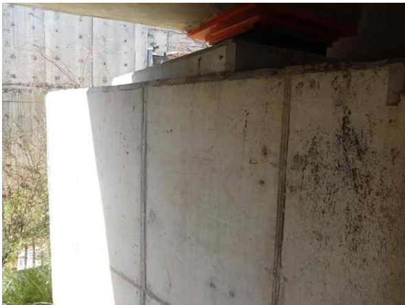
A1-Sh1 무수축몰탈 균열 (0.2mm/0.1m)
